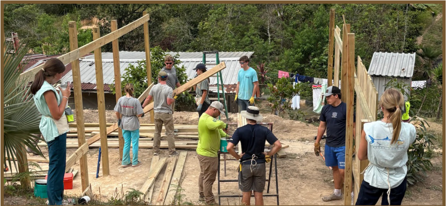
ABOVE: Youth and adult volunteers from FUMC Dothan construct the first phase of a new home which will be completed later this summer. BELOW: Measuring where to dig in order to place another post.
